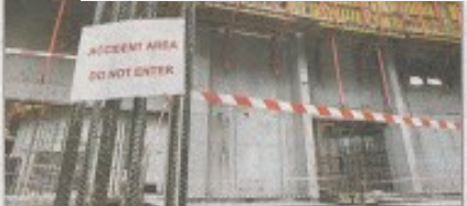
Mr Tan fell 11m to his death in this area after the ladder he was standing on wobbled while he was dismantling a wooden structure...
